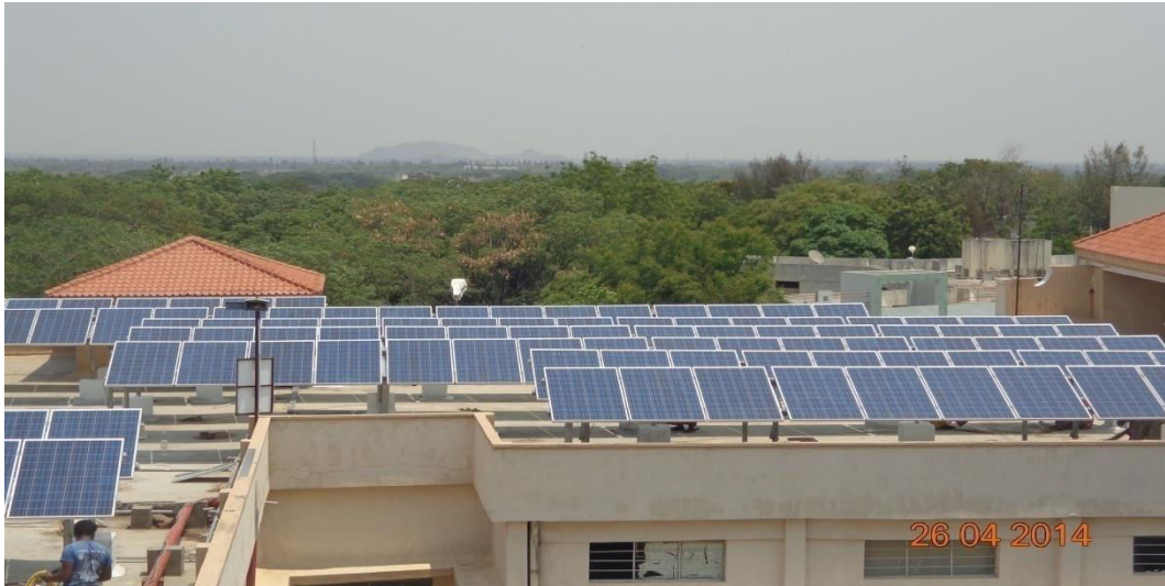
Fig- Roof Top Solar Energy Generation system
